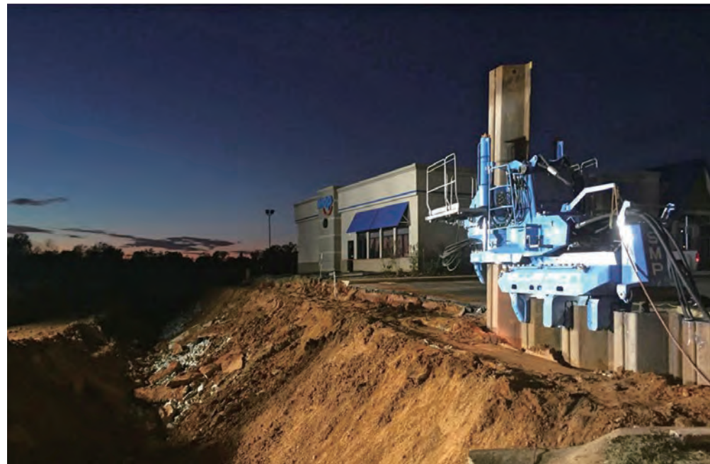
Top: After Parking Lot Collapse Bottom: Sheet Piling
