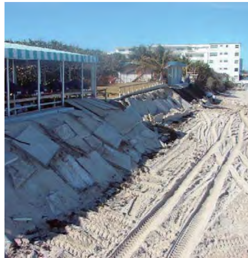
Erosion Damage (Before Construction)
