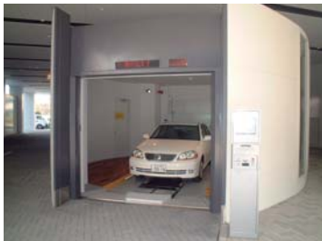
Car Park 1 exit (drive-through system)
